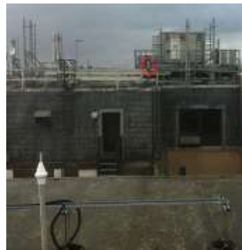
Repeating antenna is circled in red with GPS antenna in foreground
